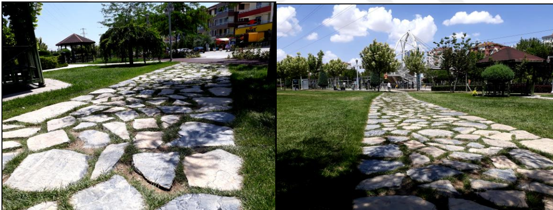
Figure 2.20 Gaps between paving materials, Konya (Personal archive, 2018)
