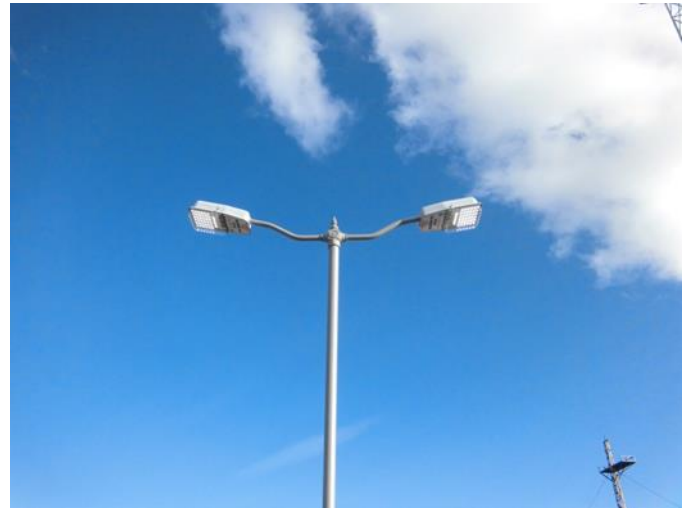
Figure 4. The streetlights used as a load
