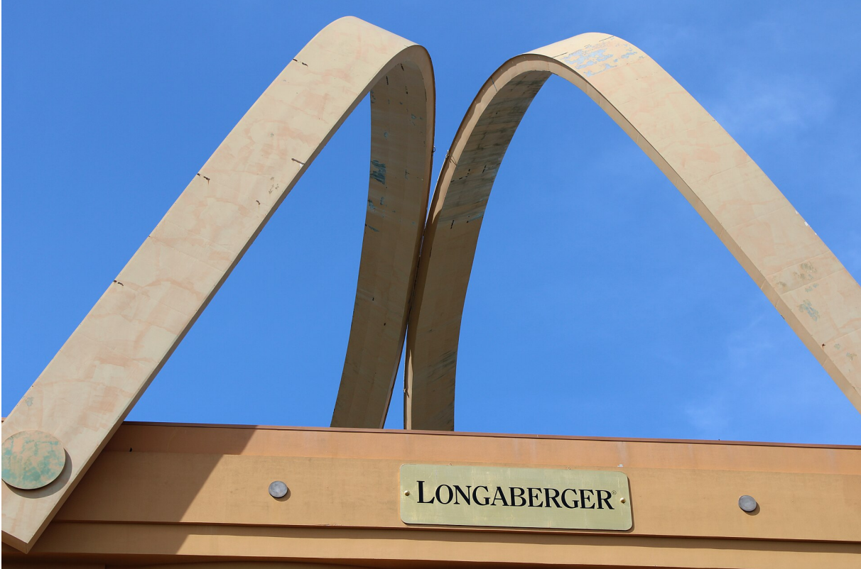
Resim 17-Longaberger Headquarters'in sepet sapları detayı. DogsRNice. (2022, Nisan). The large handles on the basket building showing signs of deterioration, building sign shown below [Fotoğraf]. Wikimedia Commons.
